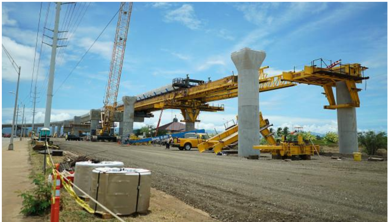
The rail guideway as it took shape in 2015 along Kualakai Parkway in Kapolei.
