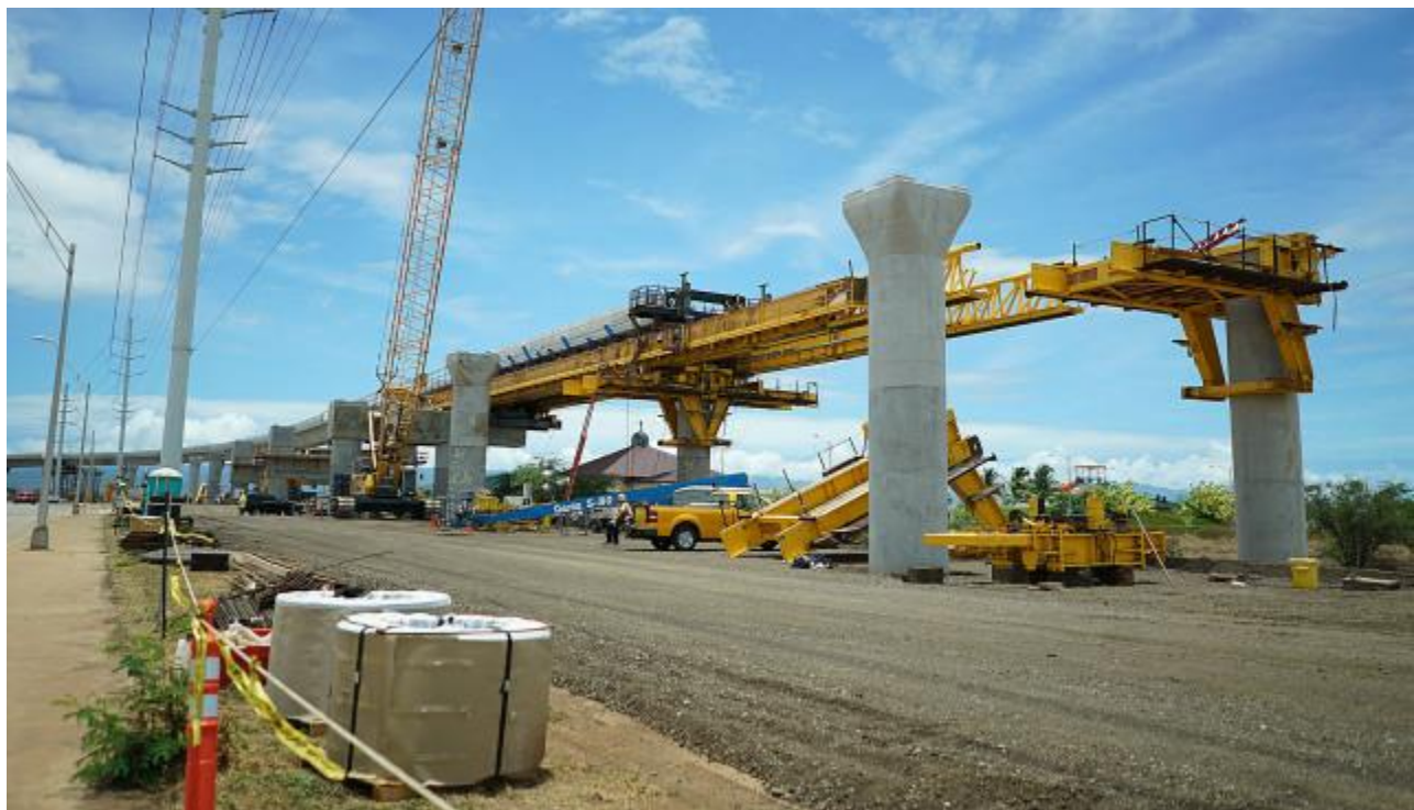
The rail guideway as it took shape in 2015 along Kualakai Parkway in Kapolei.
