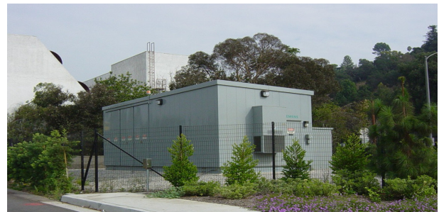
Figure 2-40 Example of a Traction Power Substation
